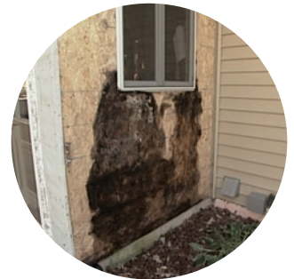
House rot from improper moisture management
