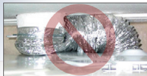
Unprotected Hose is a Fire Hazard
